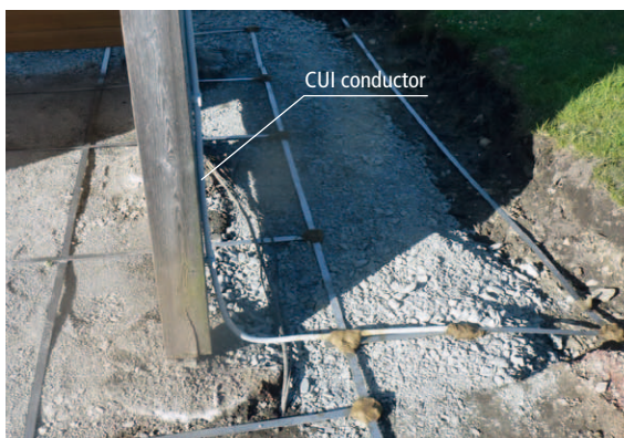
Figure 7 Practical application of an isolated lightning rod (CUI conductor)
